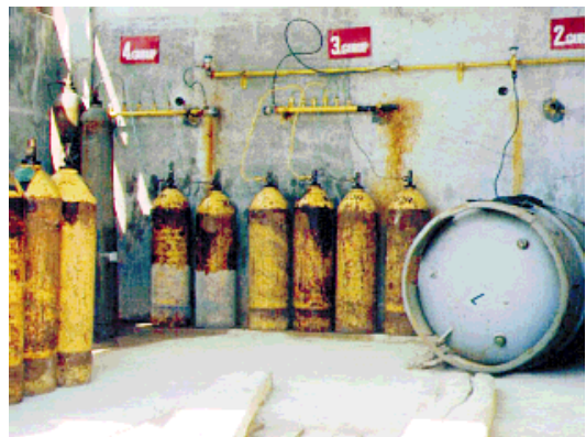
Fig. 15. Esentepe — Pumping station chlorination unit.
