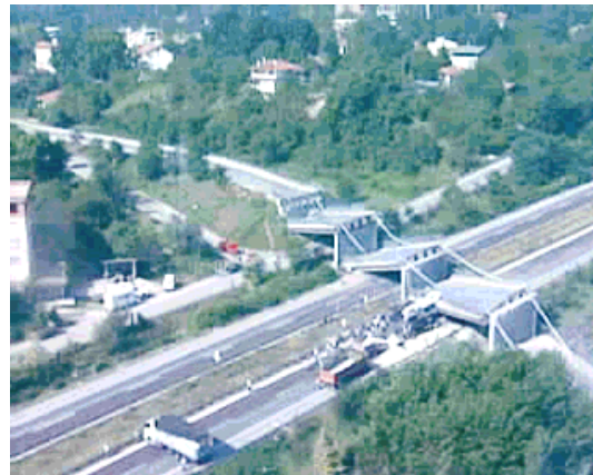
Fig. 2. Arifiye — Unseating of bridge spans at TEM overpass.
