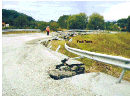
Fig. 5. Arifiye — Fault displacement effects on adjacent collectors.
