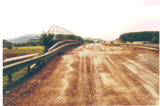
Fig. 6. Arifiye — Approach fill settlement.
