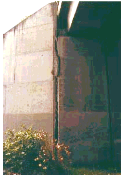
Fig. 7. Arifiye — Separation of abutment wall.
