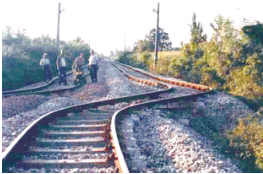
Fig. 8. Tepetarla — Temporary repair of railtrack after damage from fault offset.
