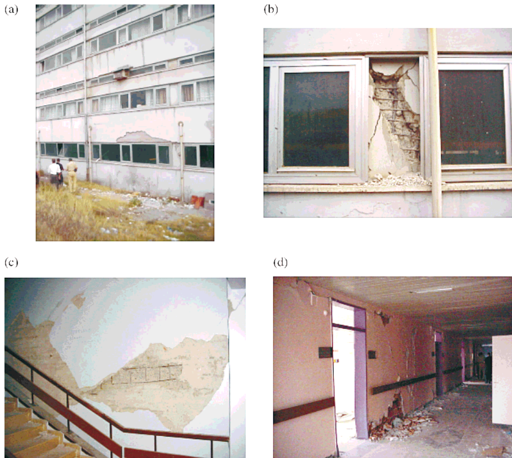
Fig. 11. Izmit — Kocaeli University Hospital: (a) elevation view of damaged nine-storey wing; (b) shear failure of 450 \times 1350 mm “short columns”; (c) shear cracking of shear wall; (d) structural and non-structural damage to partition walls.
