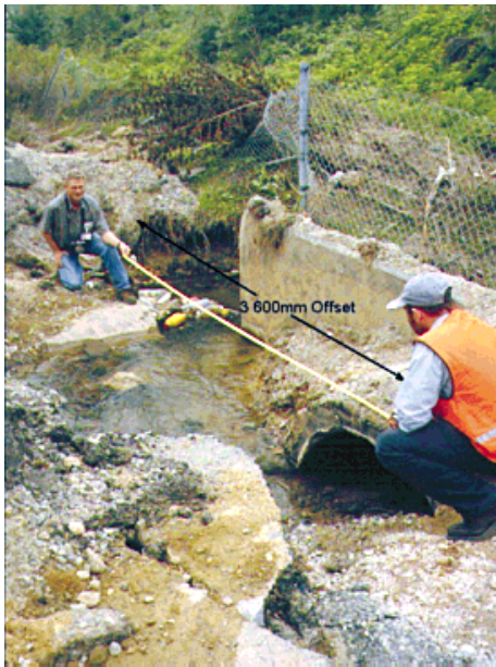
Fig. 3. Arifiye — Culvert headwall offset near overpass.
