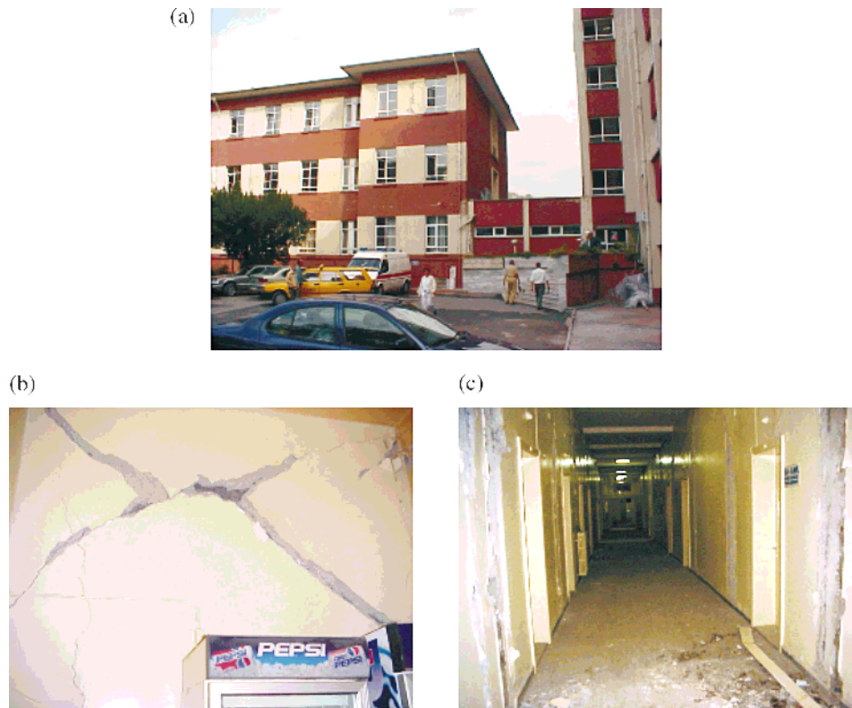
Fig. 12. Izmit — SSK Hospital: (a) general view, 1946 wing (left) and 1976 wing (right); (b) shear failure of lightly reinforced concrete wall; (c) severe damage to partition walls.
