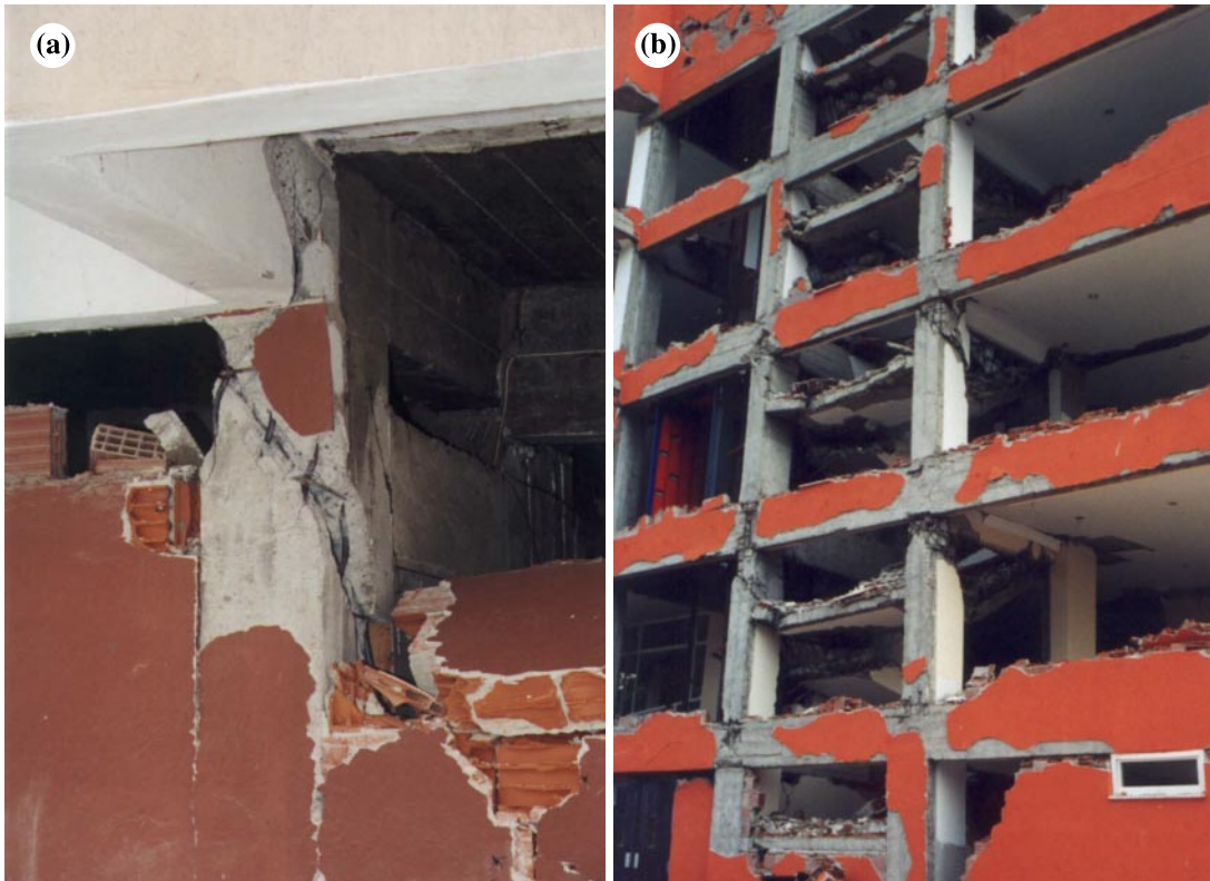
Fig. 9. Interference of non-structural elements with lateral load resisting system: (a) short column effect and (b) interference of stairway landing slabs.
