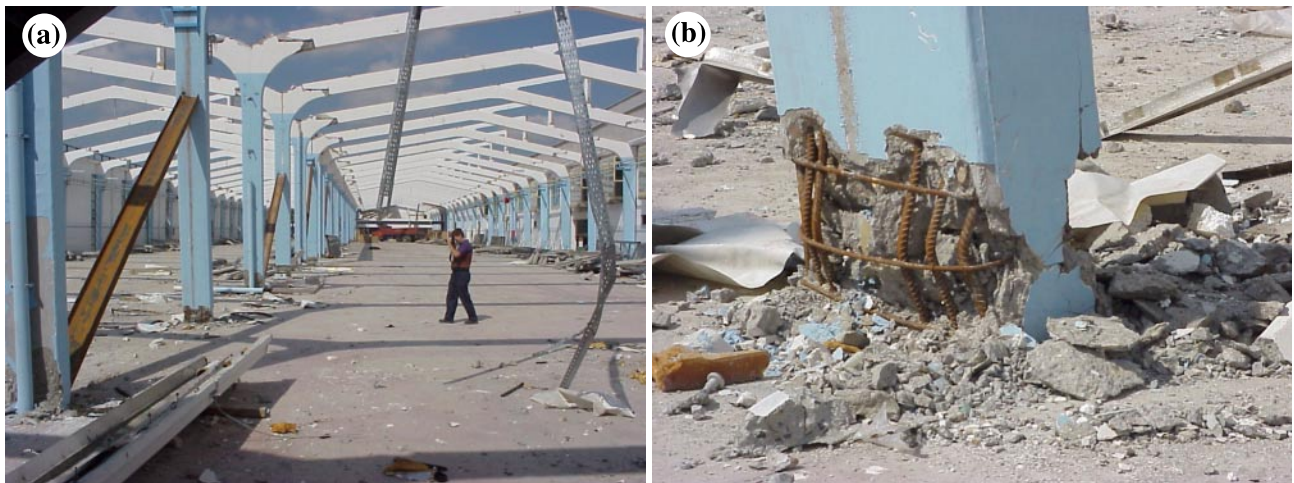
Fig. 16. Severe damage to frames of precast warehouse structure: (a) large deformation of columns and (b) flexural hinging at column base.
