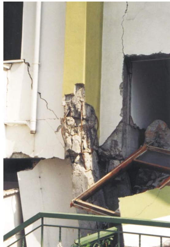
Fig. 5. Lack of transverse reinforcement in concrete columns.
