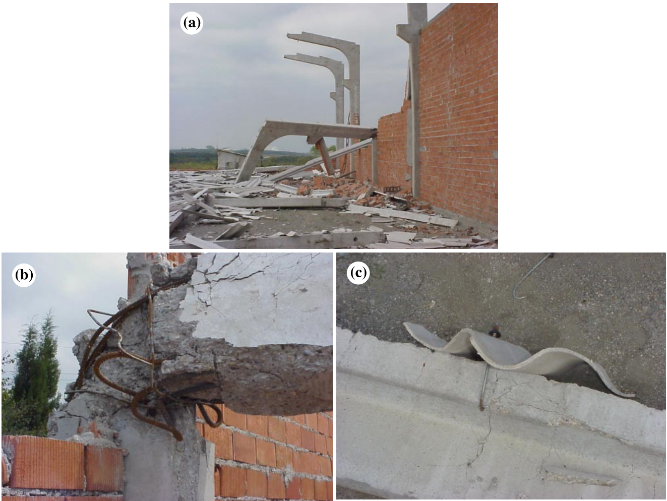
Fig. 15. Collapse of completed precast industrial building: (a) influence of partial height masonry infills; (b) inadequate confinement in columns; (c) thin corrugated fibre concrete diaphragm.
