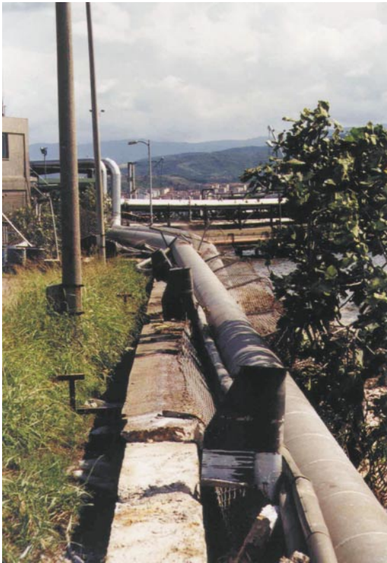
Fig. 30. Failure of pipe supports.
