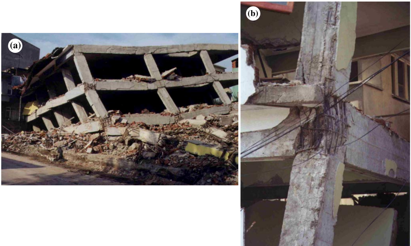
Fig. 8. Lack of joint reinforcement and resulting failures in beam–column connections.
