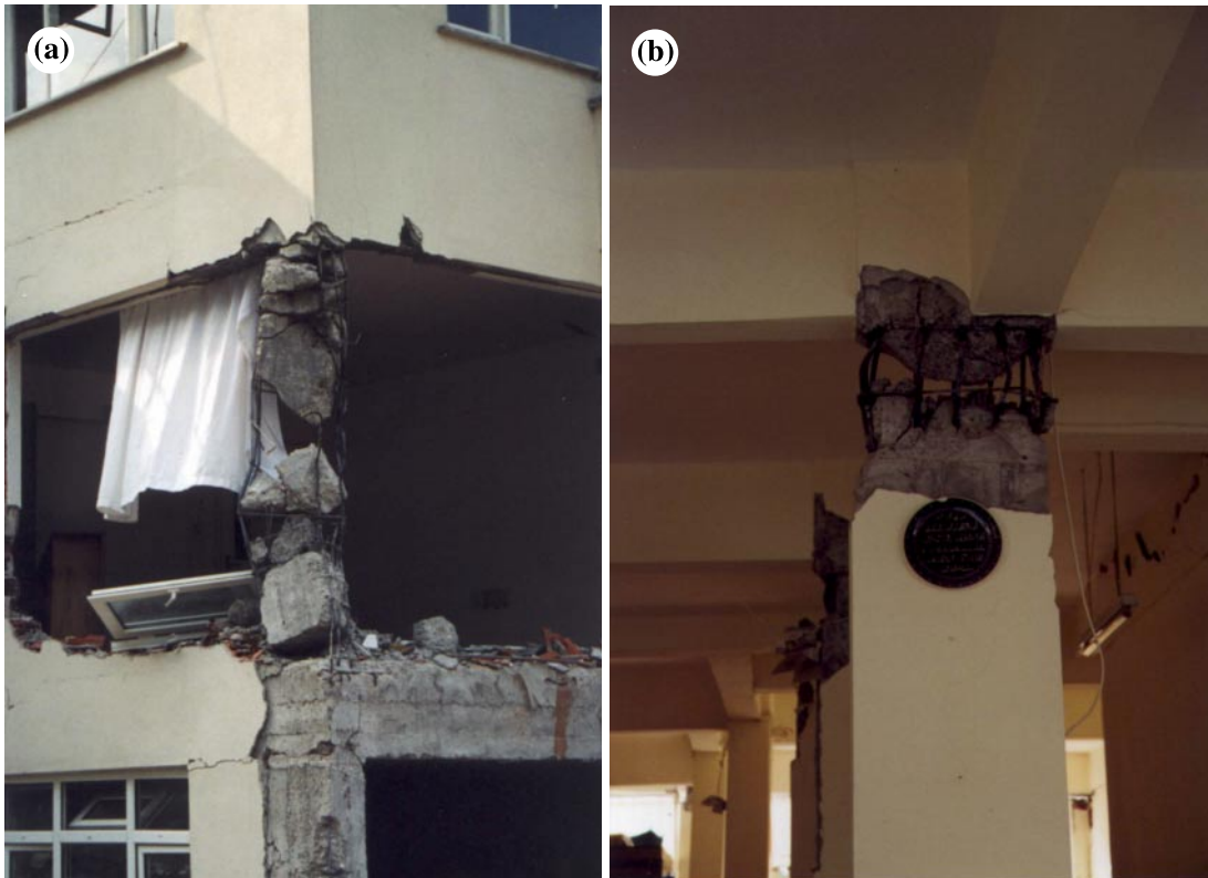
Fig. 7. Lack of column confinement reinforcement and resulting crushing.
