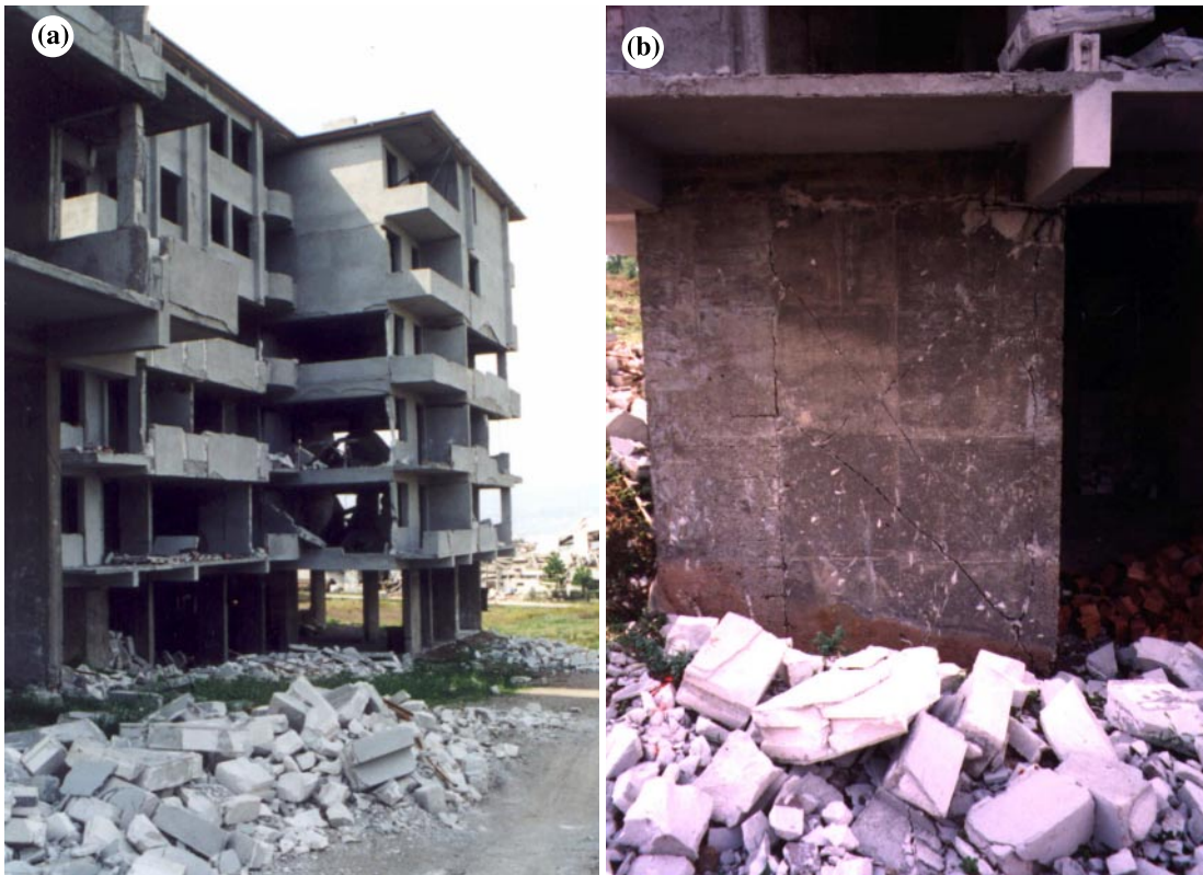
Fig. 10. Frame shear wall building with lightweight concrete masonry blocks: (a) apartment building with narrow shear walls and (b) diagonal tension cracks in shear wall.
