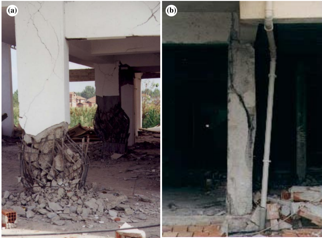
Fig. 6. Lack of transverse shear reinforcement and resulting diagonal tension failures.
