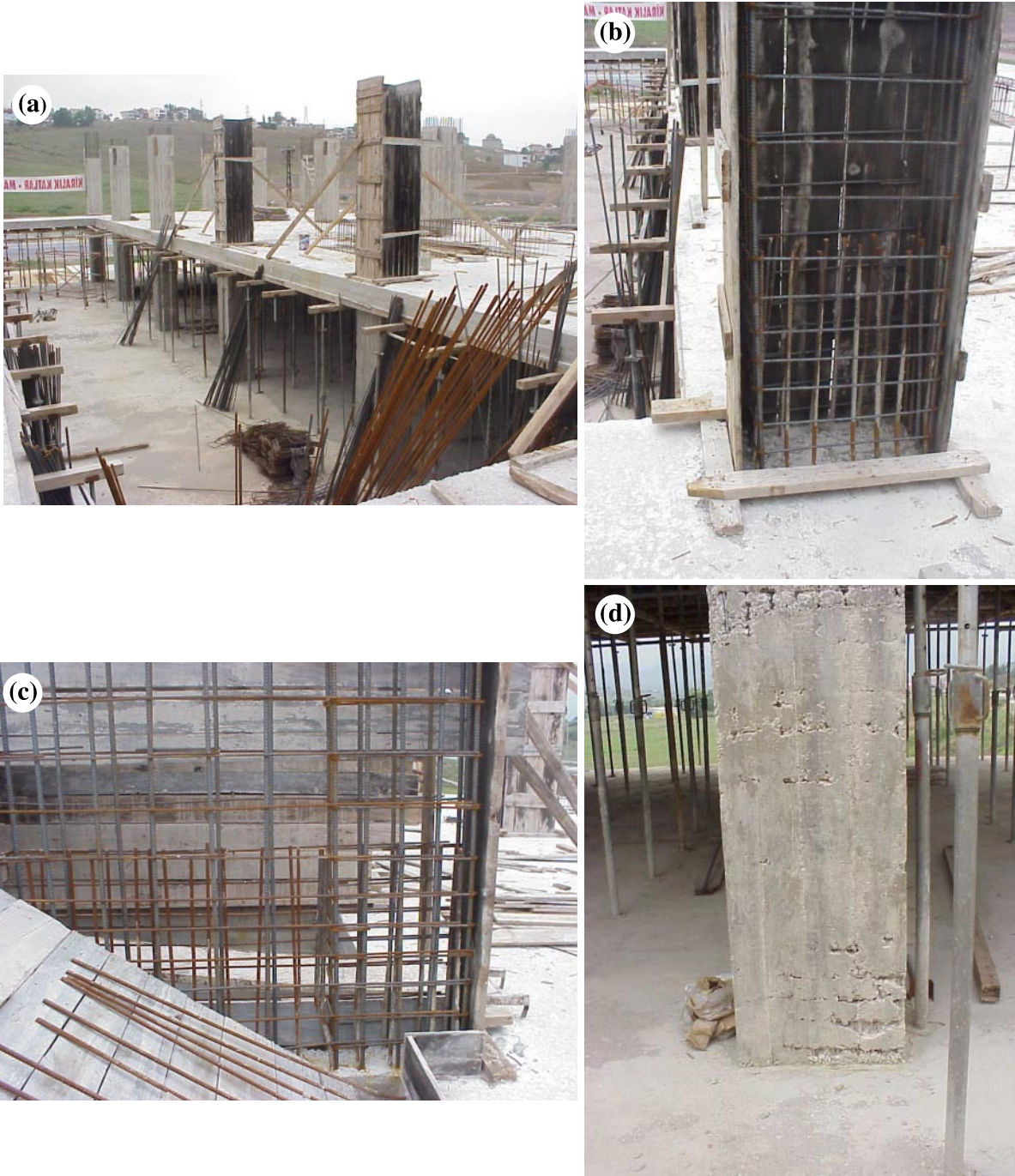
Fig. 33. Frame wall structure under construction: (a) overall view; (b) column reinforcement details; (c) wall reinforcement details; (d) insufficient concrete cover.
