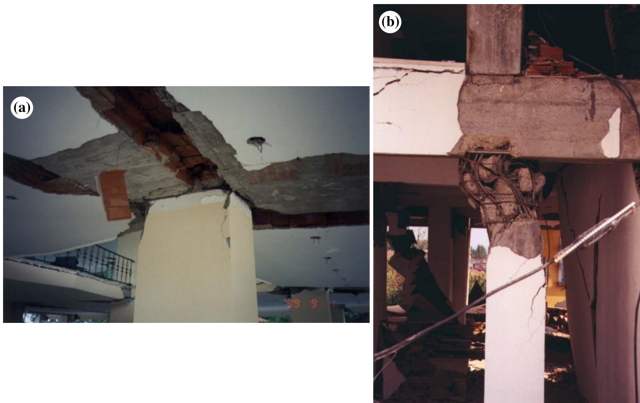
Fig. 4. Use of “Asmolen” one-way slab system and resulting strong beam and weak columns: (a) “Asmolen” concrete slab system and (b) strong-beam weak-column connection.
