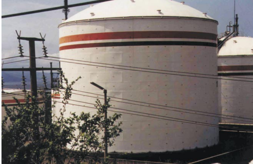
Fig. 27. Elephant foot buckling of a tank wall.
