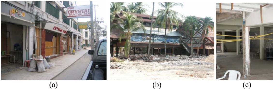
Fig. 6 Observed damage in Patong Beach
