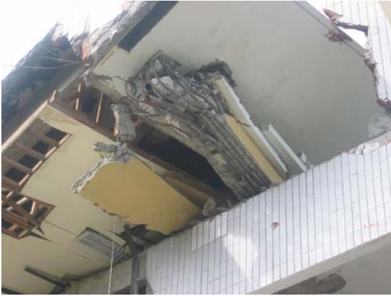
(a) Column failure in Tax Office
