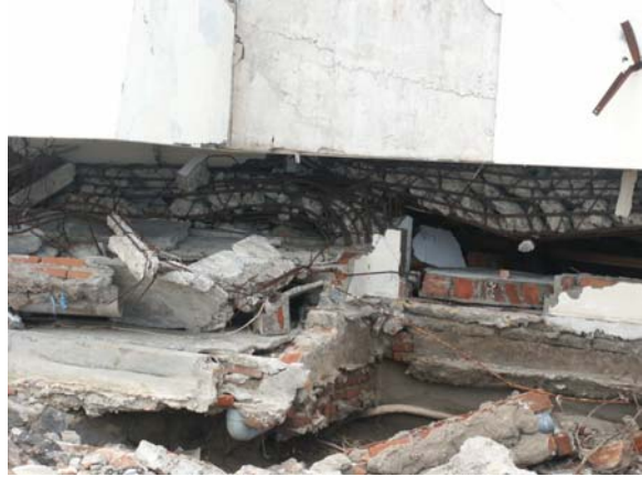
(b) Column failure in Customs Building
