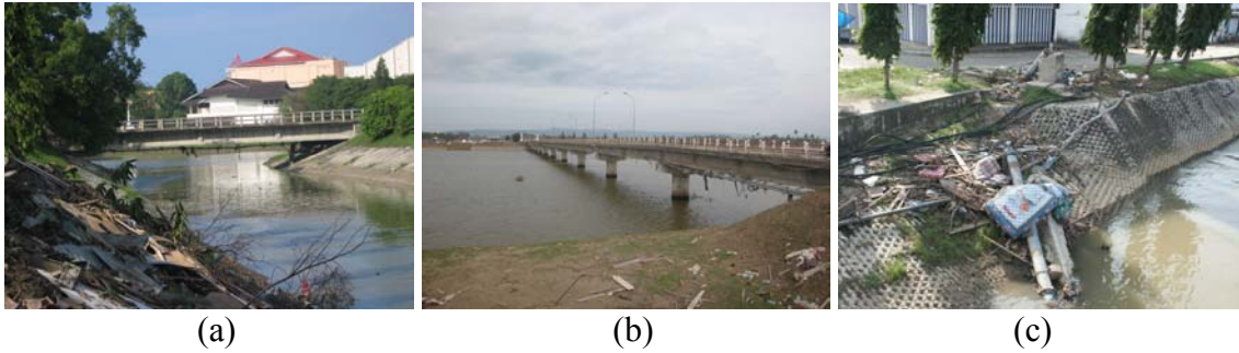
Fig. 25 Damage to pipeline attached to bridges in Banda Aceh
