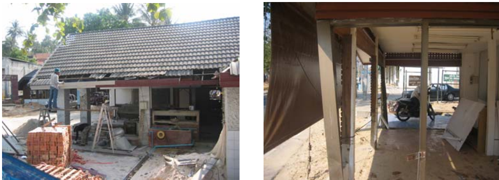
Fig. 5 Damage to single story non-engineered buildings in Kata Beach
