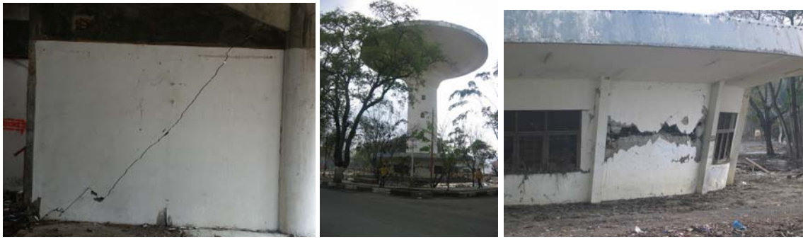
(a) Diagonal crack in a shear wall (b) Water tower (c) Shear wall at the base of tower
