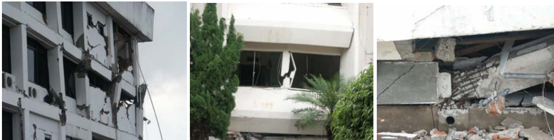
(a) Column shear failure (b) Column shear failure (c) Splice failure
