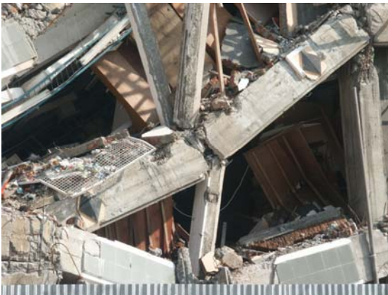
(a) Failure of beam-column connections
