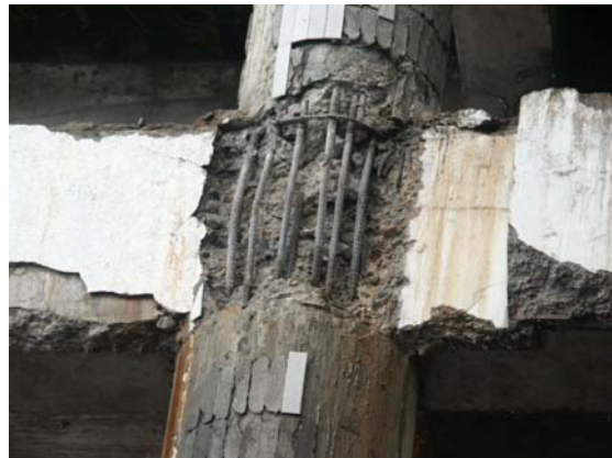
(b) Lack of joint reinforcement
