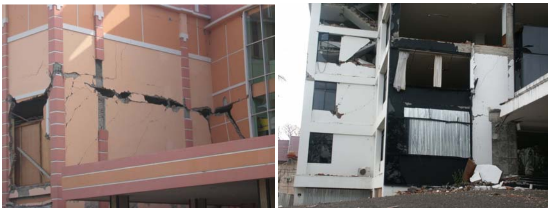
(a) Sliding shear failure (b) Diagonal tension failures
