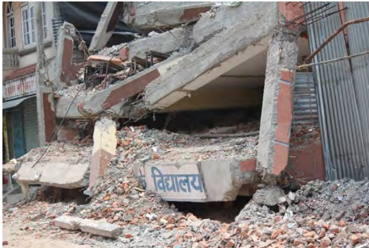
Figure 7.9: Pancake collapse of reinforced concrete building at DipJyoti Secondary School, Kathmandu
