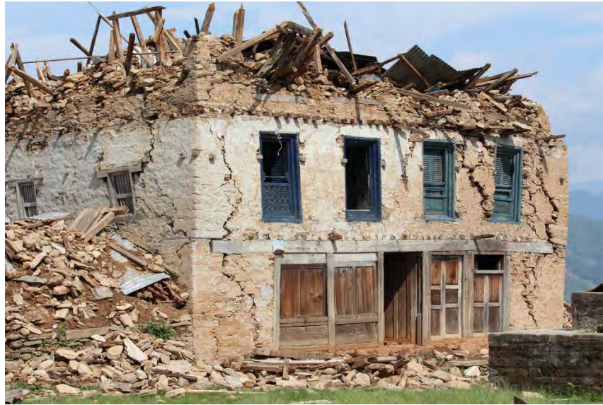
Figure 6.13: A building with floor joists bearing over the entire wall thickness (Photo: B. Pandey)
