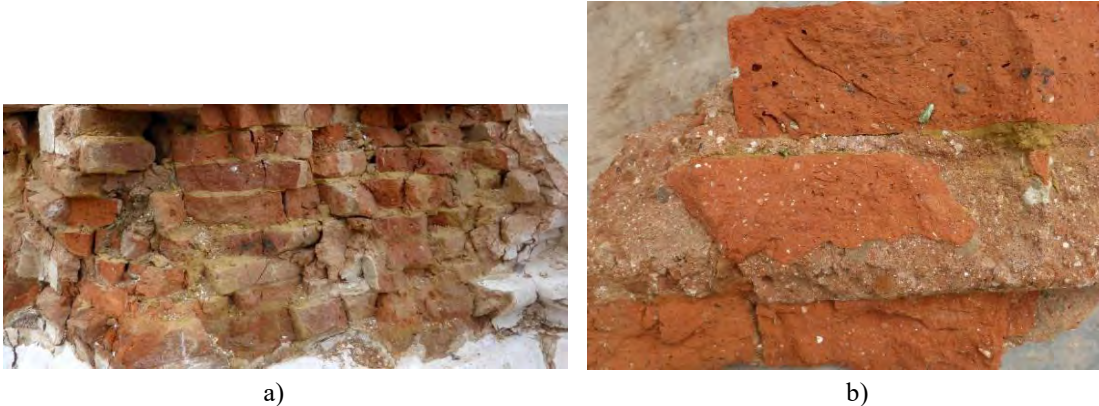
Figure 8.9: Exposed masonry construction at Pratappur temple: a) brick masonry in mud mortar at the plinth level and b) brick masonry in the lime surkhi mortar (S. Brzev)
