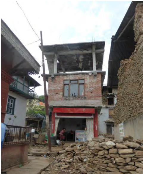
b) No visible damage to non-ductile RC frame with infill adjacent to a heavily damaged stone masonry house
