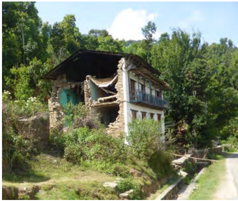
a) Complete failure of side wall
