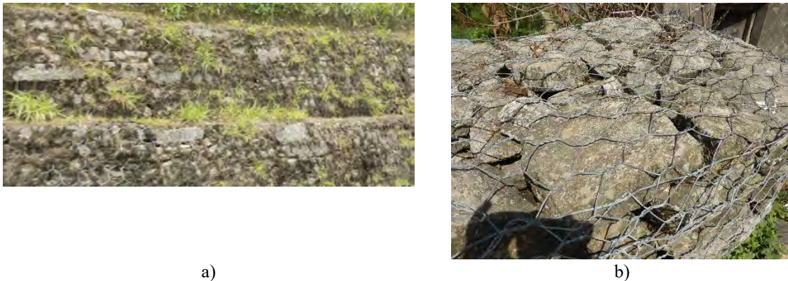
Figure 6.21: Gabion wire: a) a 30-year old application in 30-year old retaining walls in Nepal and b) a detail of the wire mesh (Photo: B. Pandey)
