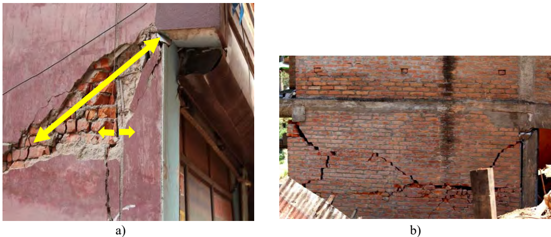
Figure 5.20: Examples of RC frame and wall interaction: a) a vertical separation crack between wall and the RC column and a diagonal shear crack extending from the wall into the column and b) in-plane shear cracking of the wall extended into adjacent RC columns (photos: Bishnu Pandey)
