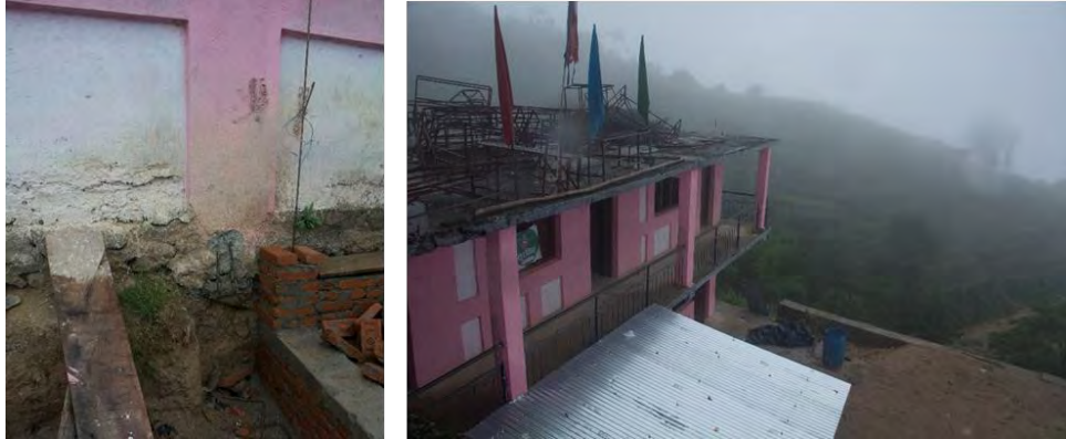
Figure 7.4: Several design and construction flaws observed in a recently upgraded school building in Kathmandu
