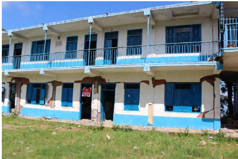
Figure 7.8: Heavy damage in Jana-Jagriti School, Sangachowk, Sindhupalchowk
