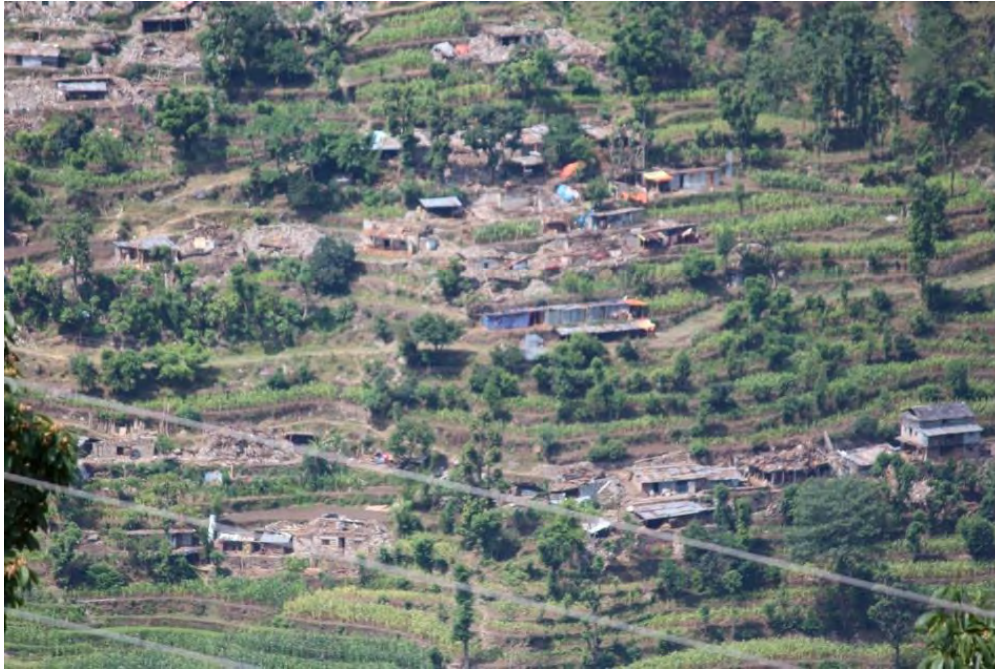
Figure 6.5: Extensive damage to rural stone masonry houses, Sindhupalchowk District (Photo: B. Pandey)
