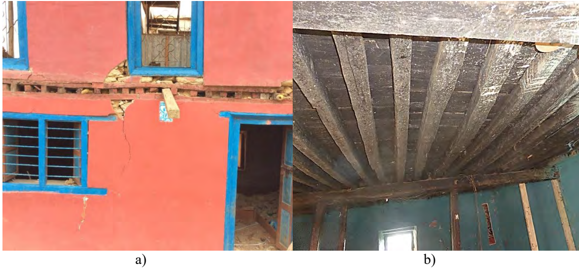
Figure 6.3: Floor structure in stone masonry houses: a) exterior view and b) interior view (Photos: S. Brzev)
