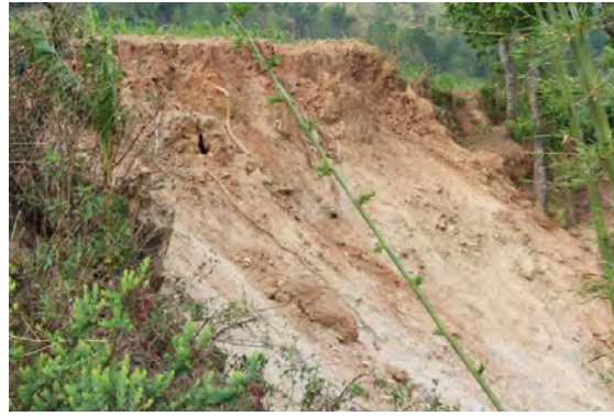
Figure 3.21: Soil failure, Dolakha District June 19, 2015 (credit: B. Pandey)
