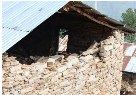
d) Failure of gable wall
