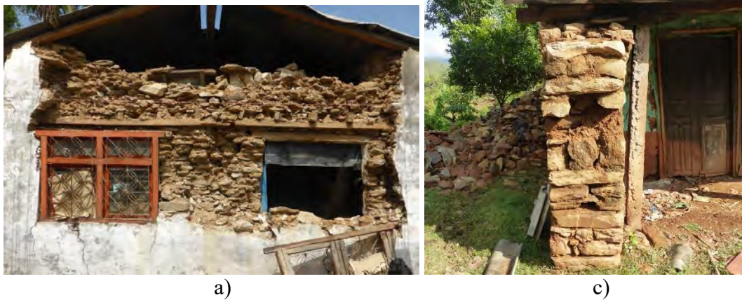
Figure 6.7: Delamination of stone masonry walls: a) an example of delamination, and b) through-stones provided in this wall are effective in preventing delamination (Photo: B. Pandey).
