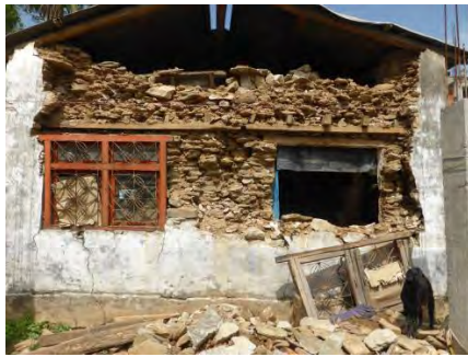
c) Failure of gable wall extended
