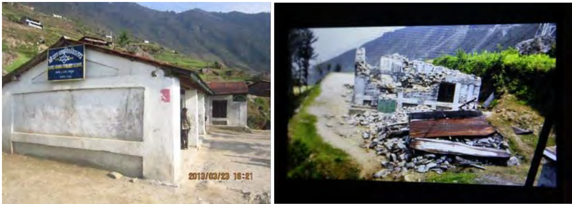
Figure 7.5: Complete collapse of retrofitted school building in Rasuwa
