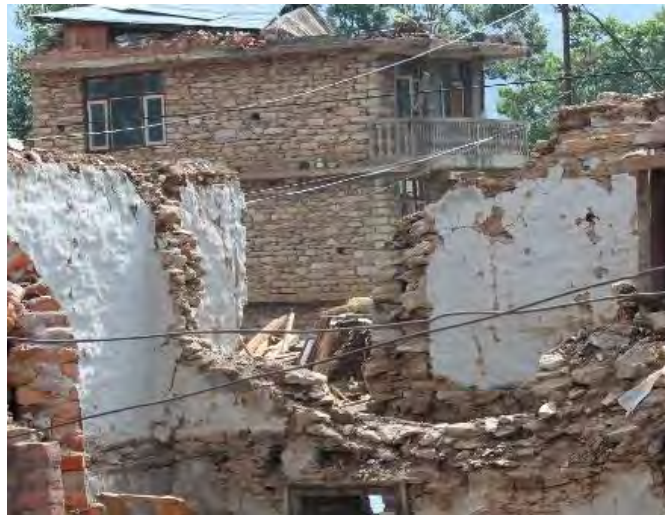
Figure 6.17: A positive effect of RC floor slabs in a stone masonry house (Photo: B. Pandey)
