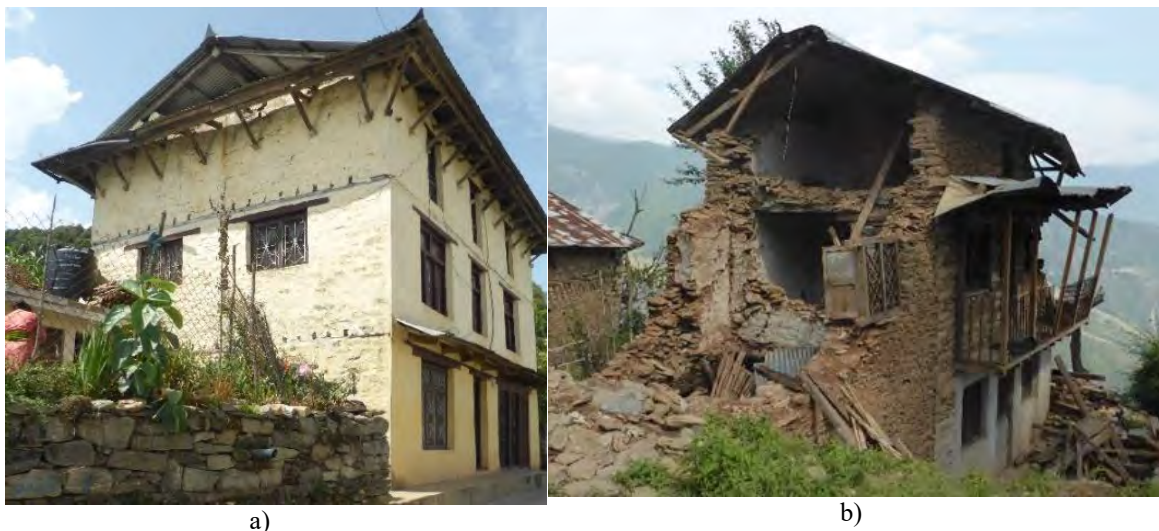
Figure 6.9: Out-of-plane failure wall collapse: a) collapse of a gable wall in an otherwise undamaged building and b) complete collapse of a transverse wall (Photos: B. Pandey)
