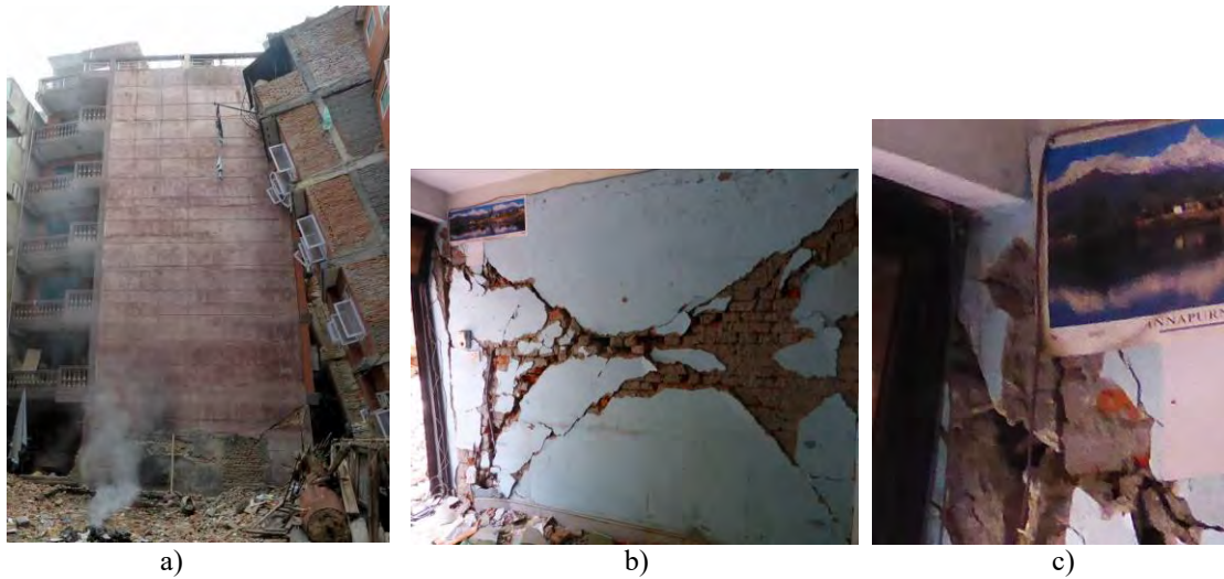
Figure 5.19: Shear failure of a RC frame building with masonry infills in the Gongobu area of Kathmandu: a) an exterior view of the building in longitudinal direction, b) an interior transverse wall showing in-plane diagonal shear failure of masonry walls, and c) diagonal cracks extended into the RC columns (photos: Svetlana Brzev)
