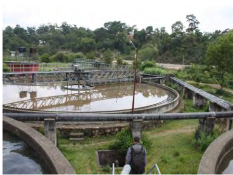
Figure 3.16: Secondary clarifiers June 14, 2015
