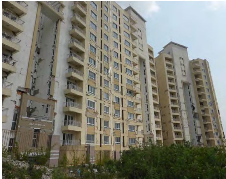
Figure 5.21: Medium-rise RC apartment building complex that experienced damage in the earthquake (photo: Svetlana Brzev)
