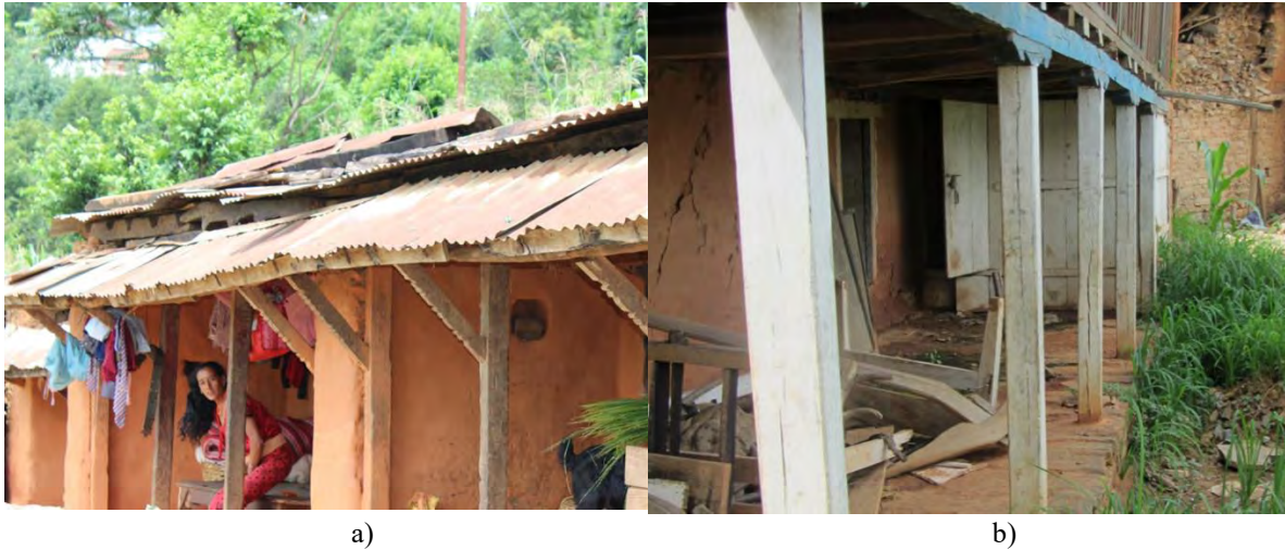
Figure 6.14: Good seismic performance of two-storey stone masonry houses: a) ground floor of a two-storey house with a porch and b) a two-storey house with a balcony (Kalikasthan village, Rasuwa District) (Photos: B. Pandey)
