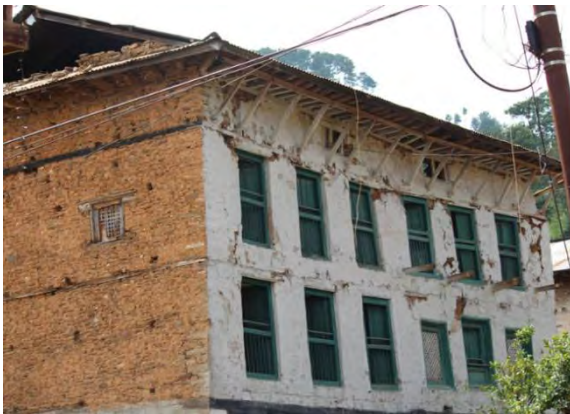
c) A stone masonry house with a large number of windows remained undamaged due to the presence of floor bands (Bhimsen).
