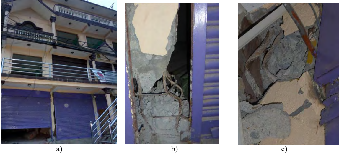
Figure 5.17: A building with an open storefront with the “weak column-strong beam” failure mechanism: a) a building elevation, b) a flexural hinge at the base of the column, and c) a flexural hinge at the top of the column (photos: Svetlana Brzev)
