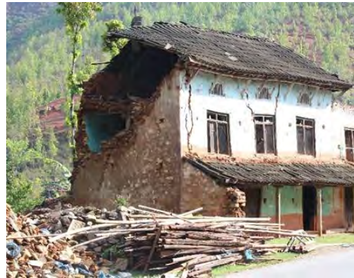
b) A partial failure of gable wall
