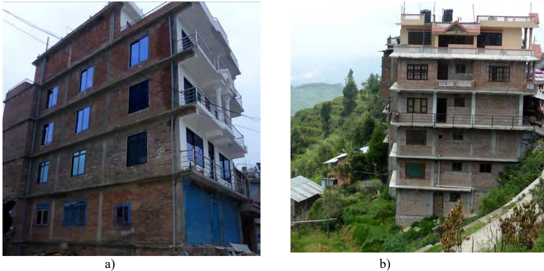
Figure 5.3: Vertical irregularities in typical low-rise RC buildings in Nepal: a) building with a setback at the top floor level and b) a building on sloped ground in a hilly area (Photos: Svetlana Brzev)
