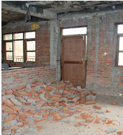
Figure 7.7: School building in Bhaktapur (Kathmandu Valley) experienced only moderate shaking, but it was deemed unsafe.
