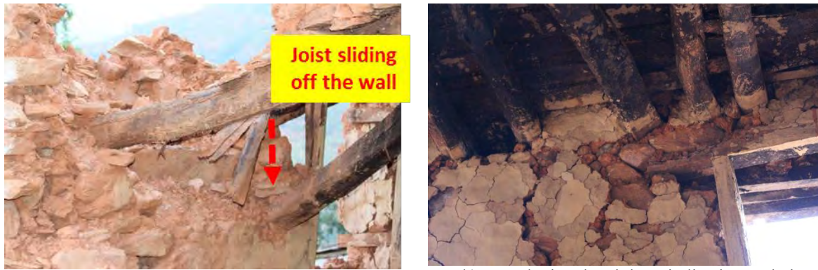
a) Floor joist about to slide off the wall
