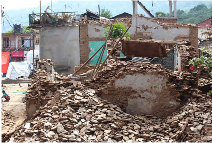
a) Extensive damage/collapse of stone masonry houses
