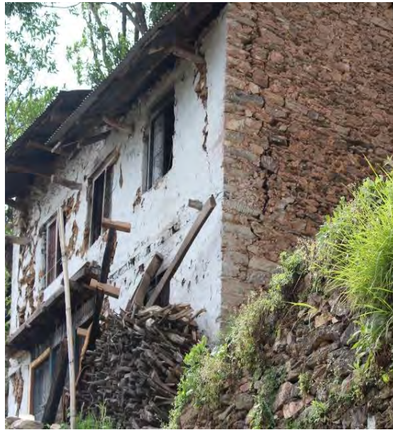
Figure 6.16: Vertical cracks in a building without timber bands (Photo: S. Brzev)
