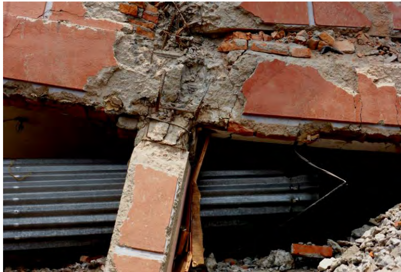
Figure 5.14: Details of a collapsed RC structure at Dipjyoti School in Kathmandu: a beam-column joint showing an absence of flexural hinging in RC beams and columns (photo: Svetlana Brzev)
