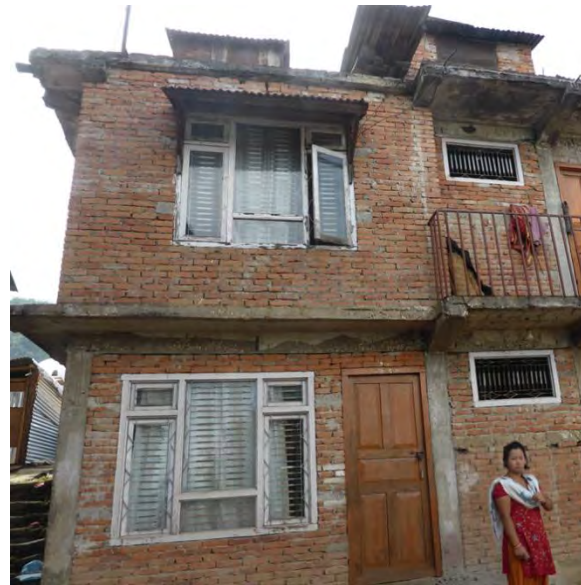
c) No damage observed in the concrete building next to damaged stone houses.
