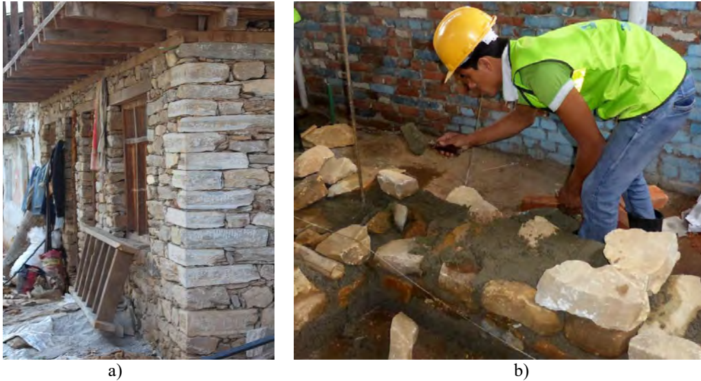
Figure 6.20: Reconstruction of stone masonry houses: a) a newly constructed stone masonry house with floor bands and corner stones and b) mason training program after the earthquake (Photos: B. Pandey and S. Brzev)
