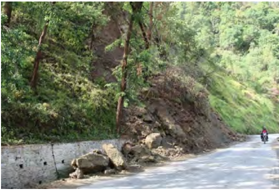
Figure 3.20: Soil failure in steep terrain June 13, 2015
