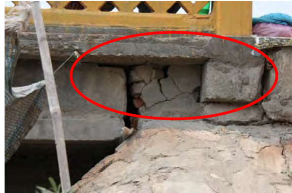
Figure 3.5: Damage to abutment June 11, 2015
