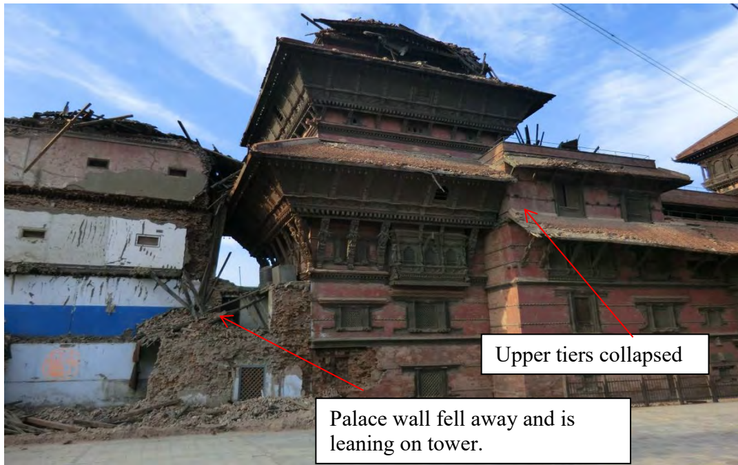
Figure 8.16: Severely damaged Basanpur Tower, Kathmandu Durbar Square (credit: David Biggs)
