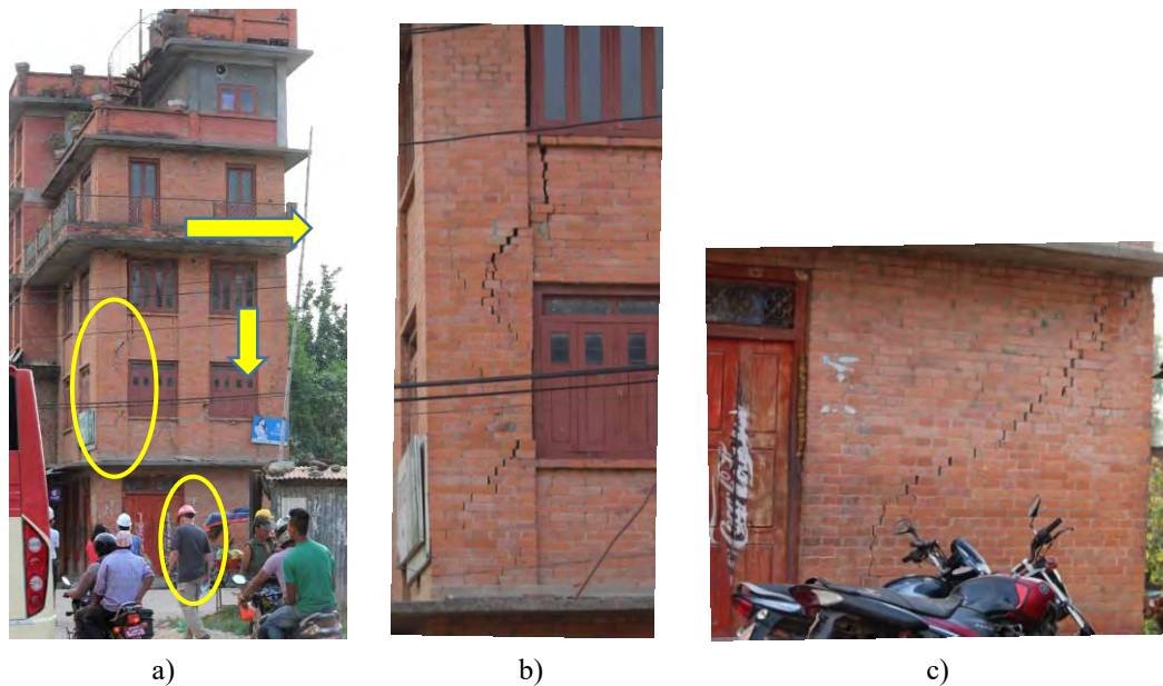
Figure 5.15: Earthquake damage due to a setback at the top storey level: a) a building elevation showing directions of lateral seismic force and compression stresses due to earthquake-induced overturning moments, b) a masonry pier showing cracks due to flexural tensile stresses and c) a wall at the base showing shear-induced diagonal tension cracks (photos: Bishnu Pandey).
