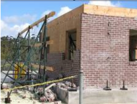
Figure 6. Collapse of Veneer on West Wall
